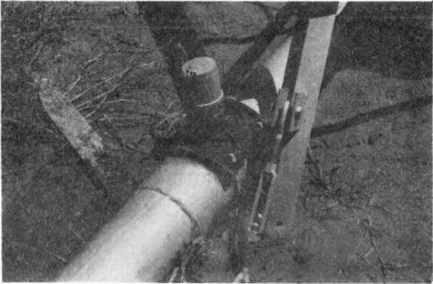
Figure 4. 8-Inch Flow Meter
